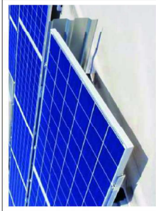
Photovoltaic Panels To Low Level Roof
